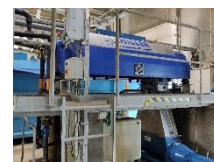
Slamafvanding i centrifuge
